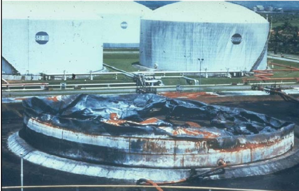
Oil refinery Pertamina, Cilacap/Java, 1995: 7 tanks burned out due to a lightning strike
